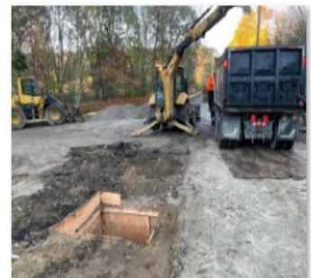
11.01.21 Well 3 Access Road.jpg
