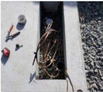
Ground cable at transformer pad.JPG
