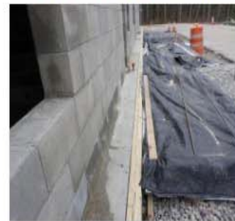
PT blocking at D-line.JPG
