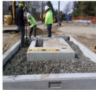
Transformer pad amd containment curb. (1).JPG
