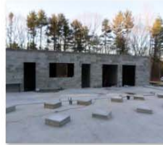
Filter tank pads 2.JPG
