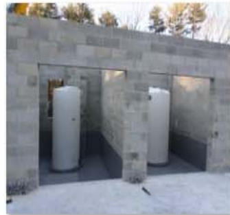
Chemical storage tanks.JPG
