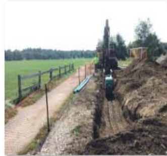
Photo 3 - Forcemain Termination Point.jpg
