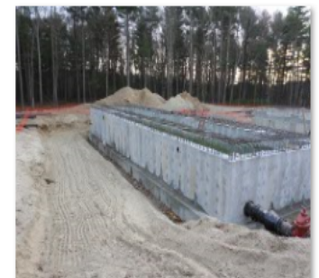
11.29.2021 Backwash Waste Tank 2.JPG
