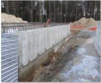
11.29.2021 Backwash Waste Tank.JPG
