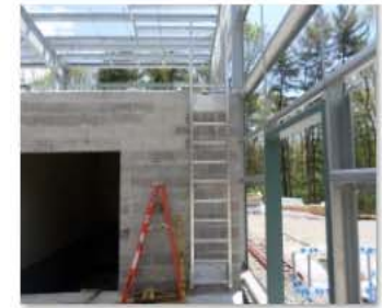
Aluminum ladder to upper level.JPG
